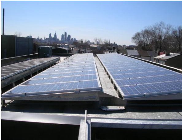
Figure 1-1: Eleven PV systems with total capacity of 26.6 kW at Rag Flats Condominiums, Philadelphia
