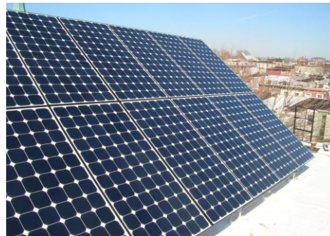
2.94 kW Rooftop PV System, Philadelphia Source: Celentano Energy Services
