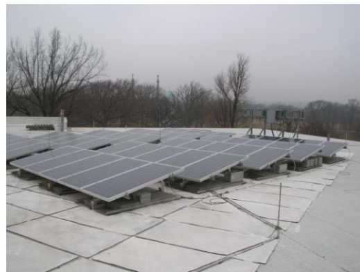
Figure 2-11: Commercial ballasted 8.5 kW PV system – Microsoft School
