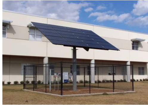
Figure 2-12: Pole-mounted PV system for a Middle School
